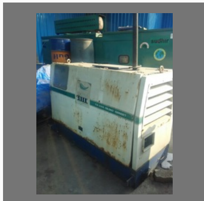
High Voltage Used Generators
