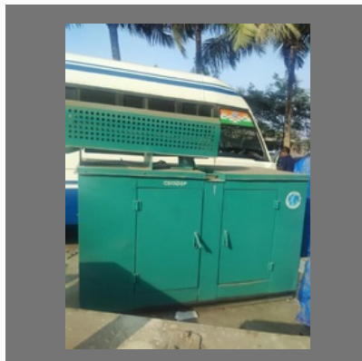
Long Life Electricity Used Generators
