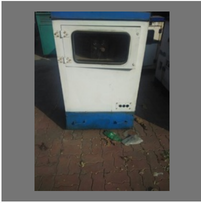
Regular Use Generator
