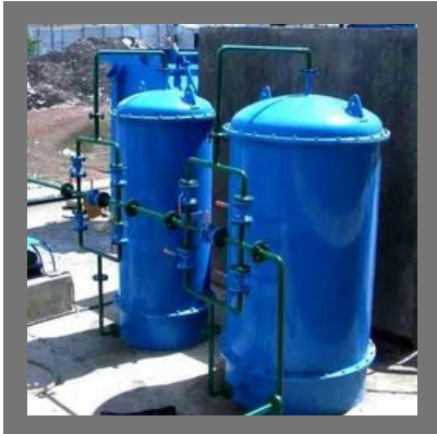
Pressure Sand Filter
