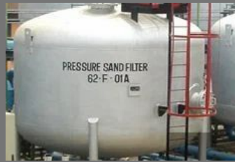
Waste Treatment Plant
