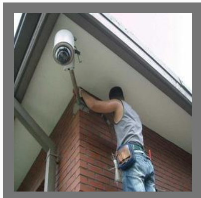
CCTV Installation Services
