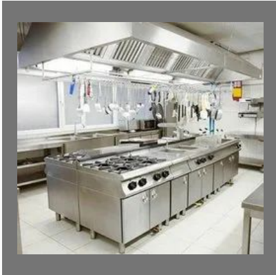
Commercial Kitchen Equipment
