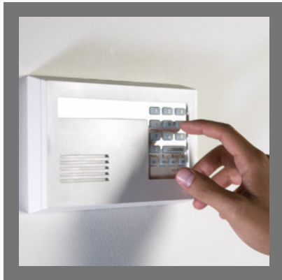
Intrusion Alarm System
