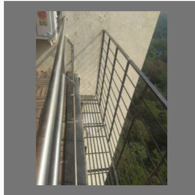
Mild Steel AC Platform With Railing
