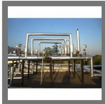
Pressure Reducing Station Fabrication Service
