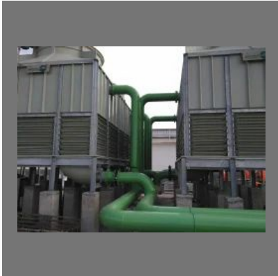
Cooling Water Piping System
