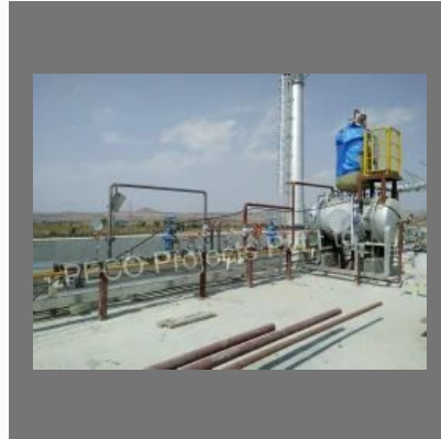
IBR Steam Piping
