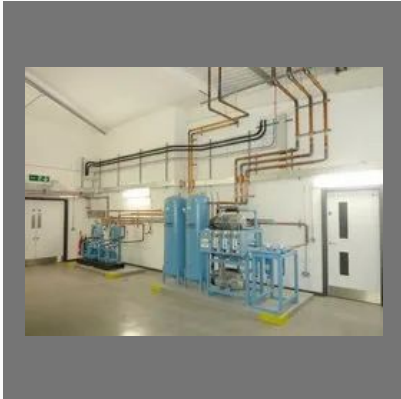
Medical Gas Pipe System
