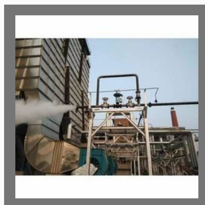
IBR Piping Services
