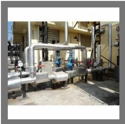
Pressure Reducing Station Turnkey Project
