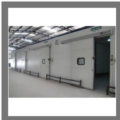
Cold Storage Automation Service
