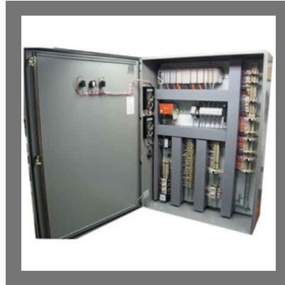
Electrical Control Panel
