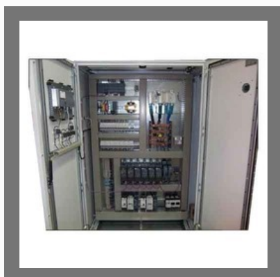
Automation Control Panel
