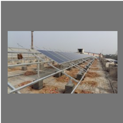
Rooftop Solar Power Plant
