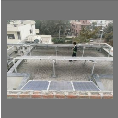
Solar Roof Top
