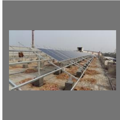
Solar On Grid System
