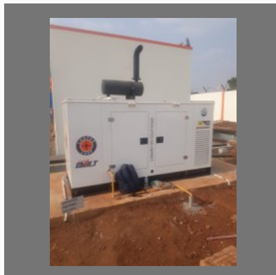
Cooper Piped Natural Gas Generator
