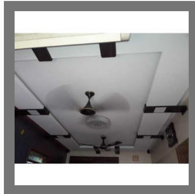
POP Ceiling Designing Service
