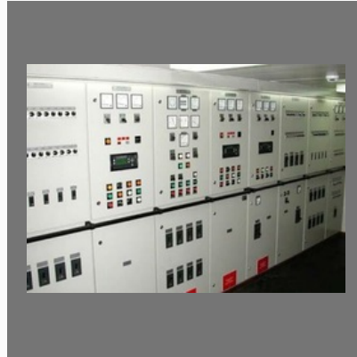
Electrical Control Panel
