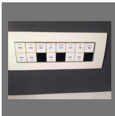
Remotely Operated Switches
