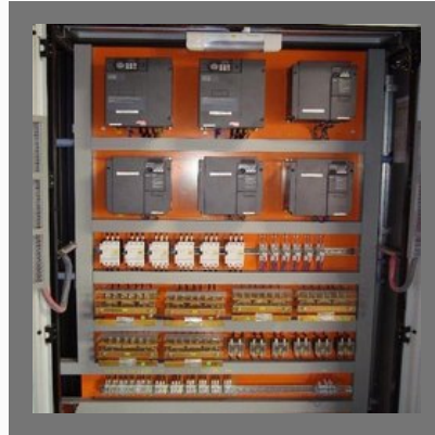
AC Drive Control Panel
