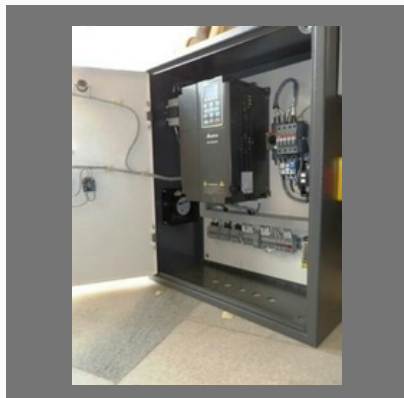
Electric Control Panel
