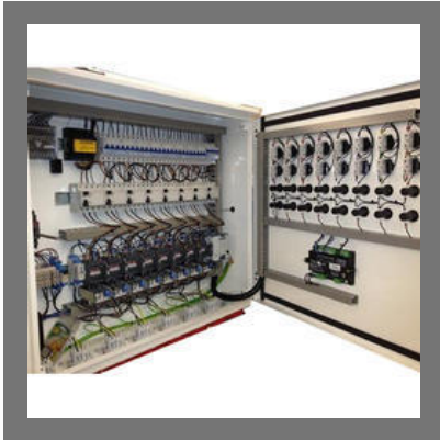
Power Control Panel
