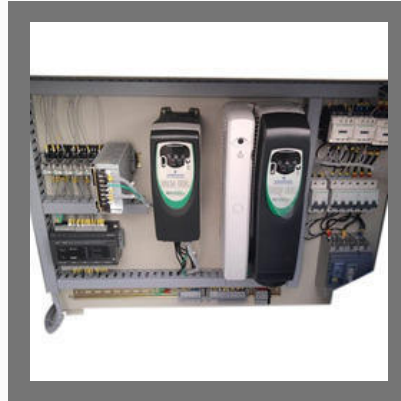
VFD Control Panel
