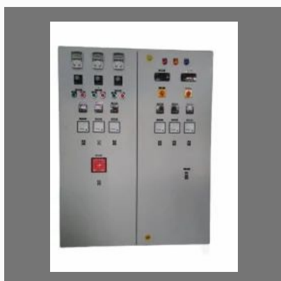
Electrical Feeder Pillar Panel
