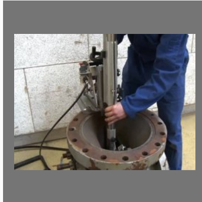
All types of Valves Servicing
