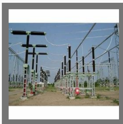
Electrical Substation Work
