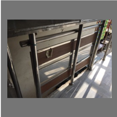
SS Wooden Staircase
