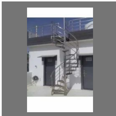
Stainless Steel Stair Railing
