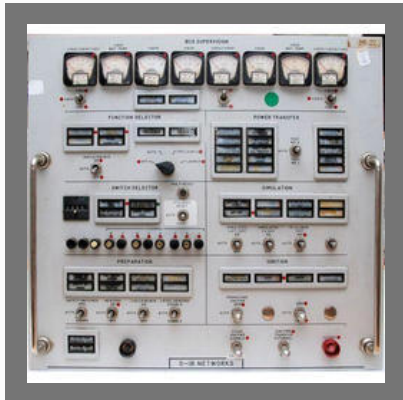
Electrical Control Panel
