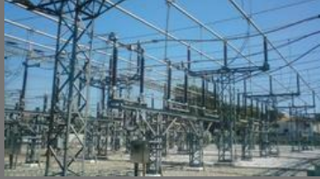
Power grid & Substation contractors
