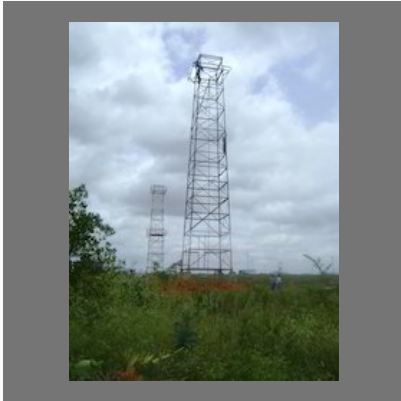
Electrical And Telecommunication Towers
