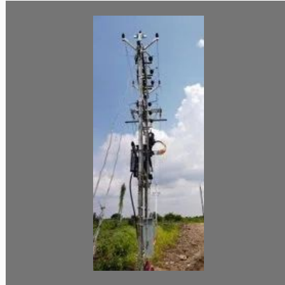
Electrical Equipment Maintenance Service
