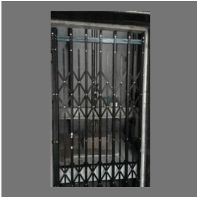
Elevator Collapsible Gate
