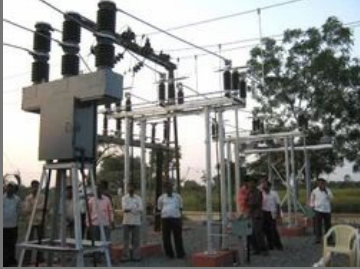
Electrical Substation Work
