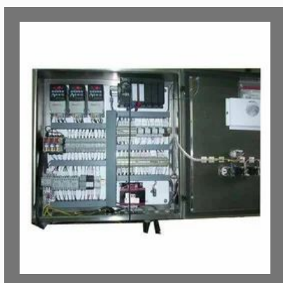
AC Drive PLC Control Panel
