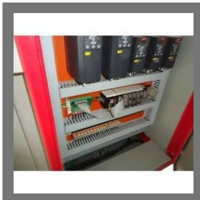
AC Drive Control Panel
