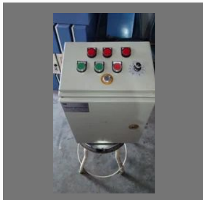
AC Drive Panel for SPM Application
