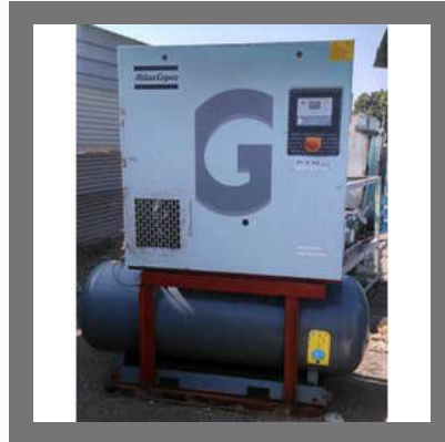
Atlas Copco Air Compressor
