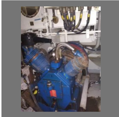
sperre air compressor
