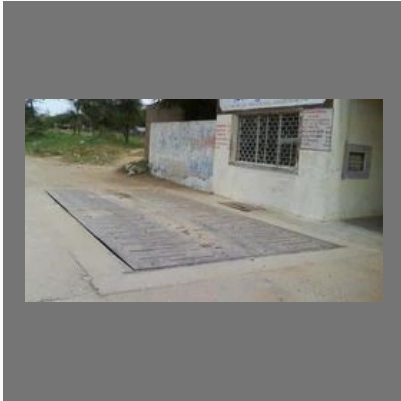
Pit Type Weighbridge
