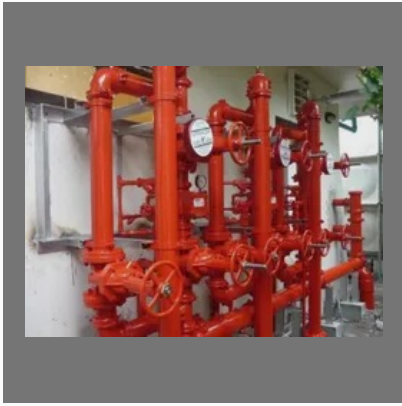
Fire Fighting System
