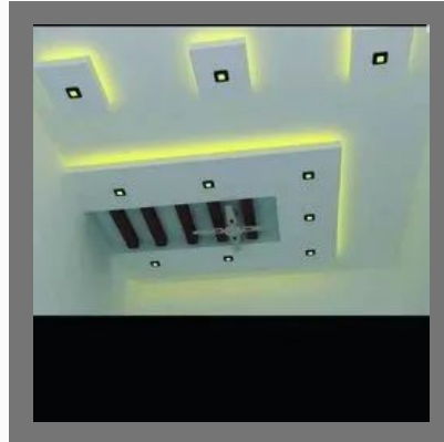
Gypsum False Ceiling
