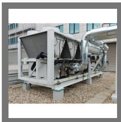
Air Cooled Chillers
