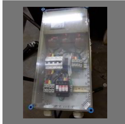
Solar GIP with Metering
