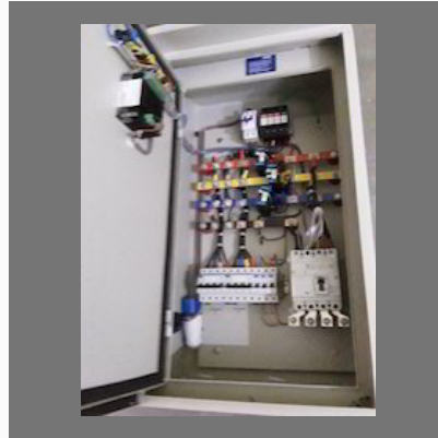
Solar ACDB - Outdoor
