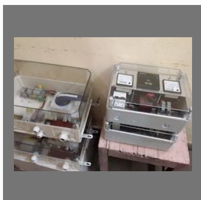
Solar AJB with DC Metering
