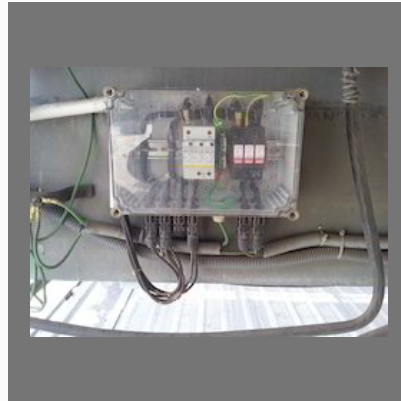
Solar Array Junction Box with SPD
