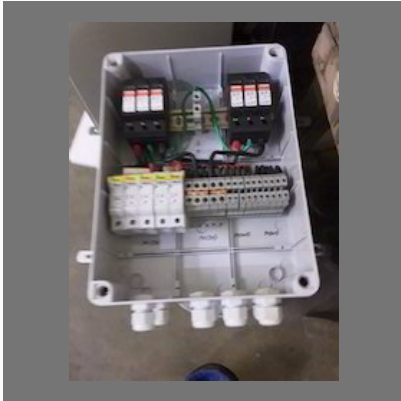
Solar Array Junction Box
