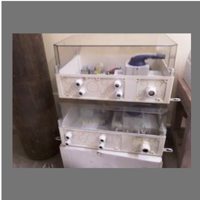
OFF Grid Solar Array Junction Box
