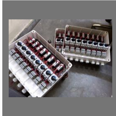
Solar Array Junction Box With DC Isolator
