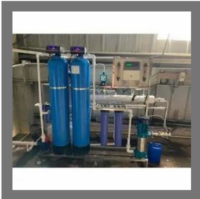
Industrial 200 LPH Reverse Osmosis Plant
