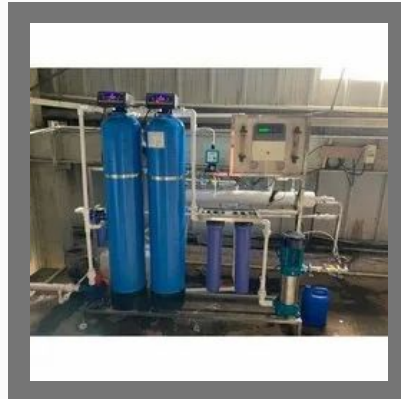
500 LPH Reverse Osmosis Plant
