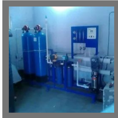
1000 LPH Reverse Osmosis System
