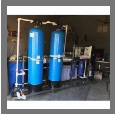
2000 LPH Reverse Osmosis Plant
