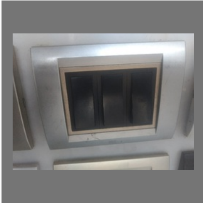
Electric Switch Board
