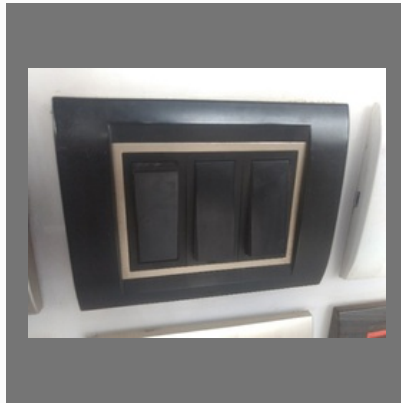
Electric Switch Board
