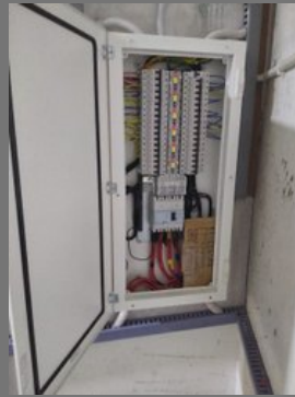
Meter Panel Board
