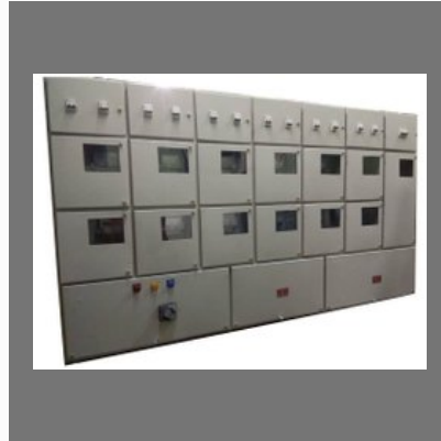
Power Distribution Panel
