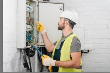
House Electrical Wiring Service
