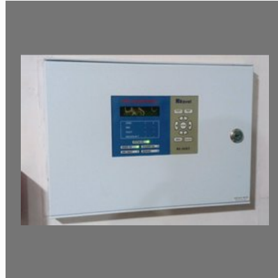
Fire Alarm System
