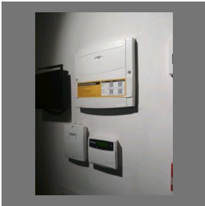
Home Automation System
