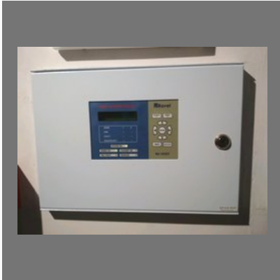
Fire Alarm System
