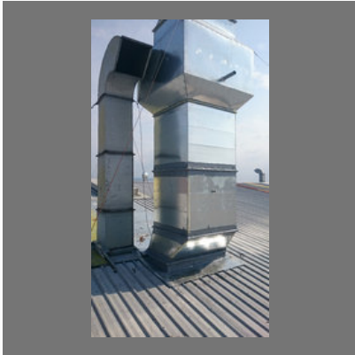
Industrial Air Duct
