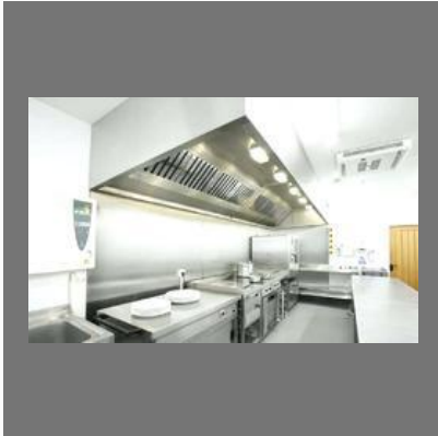
Commercial Kitchen Exhaust Hood
