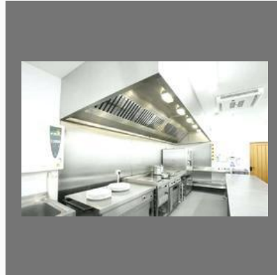
Commercial Kitchen Hood
