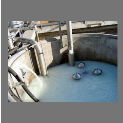
Industrial Wastewater Treatment Plants
