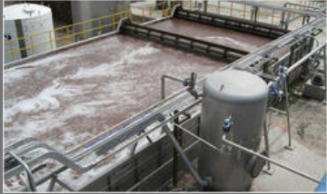
Effluent Treatment Plant Services
