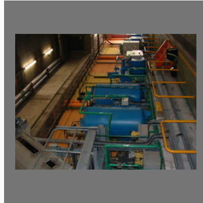
Sewage Treatment Plants
