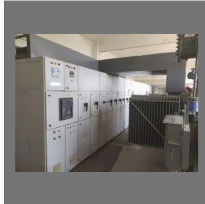
Electrical Distribution Control Panel
