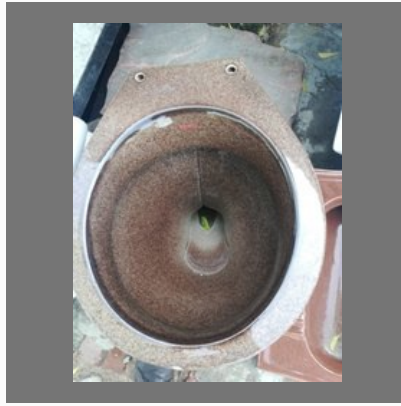
Western Style Toilets
