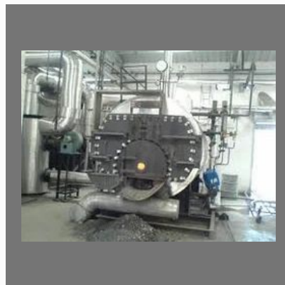
Industrial Coal Fired Boilers
