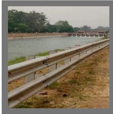
W Beam Crash Barrier
