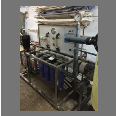
Industrial Reverse Osmosis Plant
