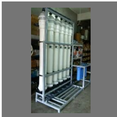
Ultra Filtration Plant
