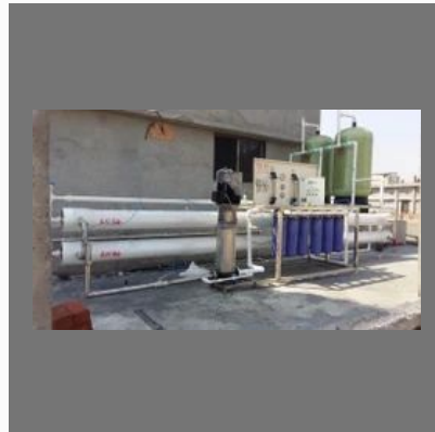
10000 Lph R.O Plant
