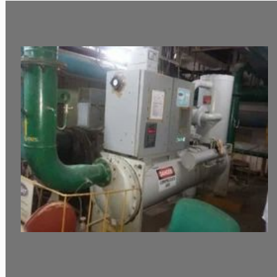
On Line Water Chillers
