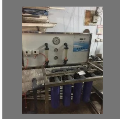
Industrial Reverse Osmosis Plant
