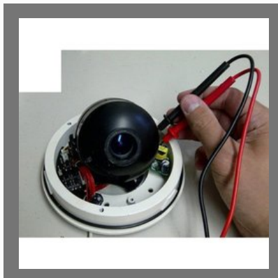
CCTV Camera AMC Service
