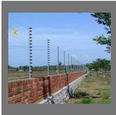
Boundary Wall Electrical Fencing
