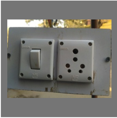
Electric Switch Board
