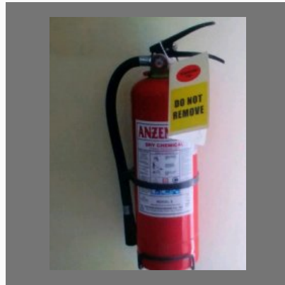
Fire Safety Equipment
