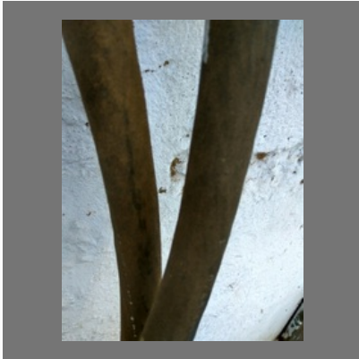
High Voltage Wires
