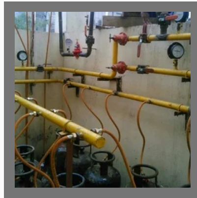
Commercial Gas Pipeline Fitting
