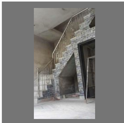
Stainless Steel Stair Railing
