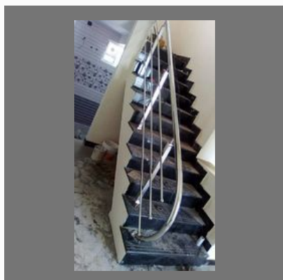
Stainless Steel Stair Railing
