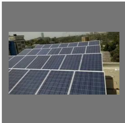
On Grid Solar System
