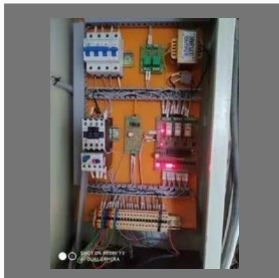
Power Distribution Panel
